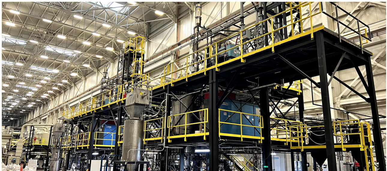
Generation 3 Furnace systems and milling equipment installed in NOVONIX's Riverside facility
