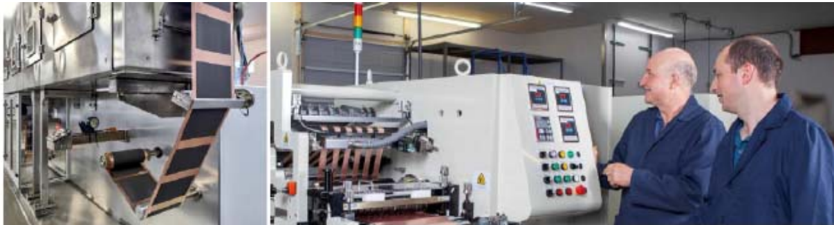
Photo: Professor Jeff Dahn and NOVONIX's COO Dr Chris Burns inspecting battery assembly at the NOVONIX pilot cell manufacturing line in Bedford (near Halifax) Nova Scotia Canada.
